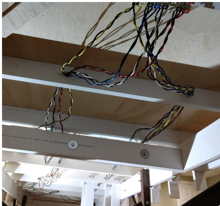
Wiring 13 – Wiring connecting all 4 terminal blocks
